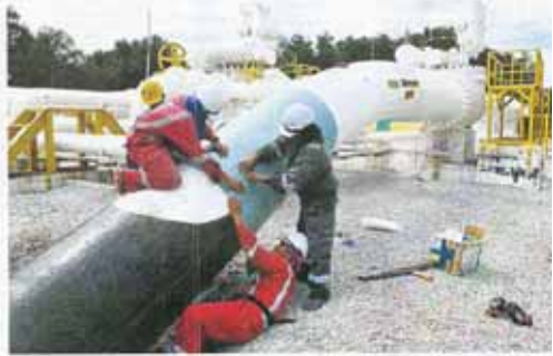
Tariff up: Contract workers patching on a gas pipe at the Kluang Porton natural gas station. From next year, the effective gas tariff rate will be increased by an average of 19%. — Bernama
