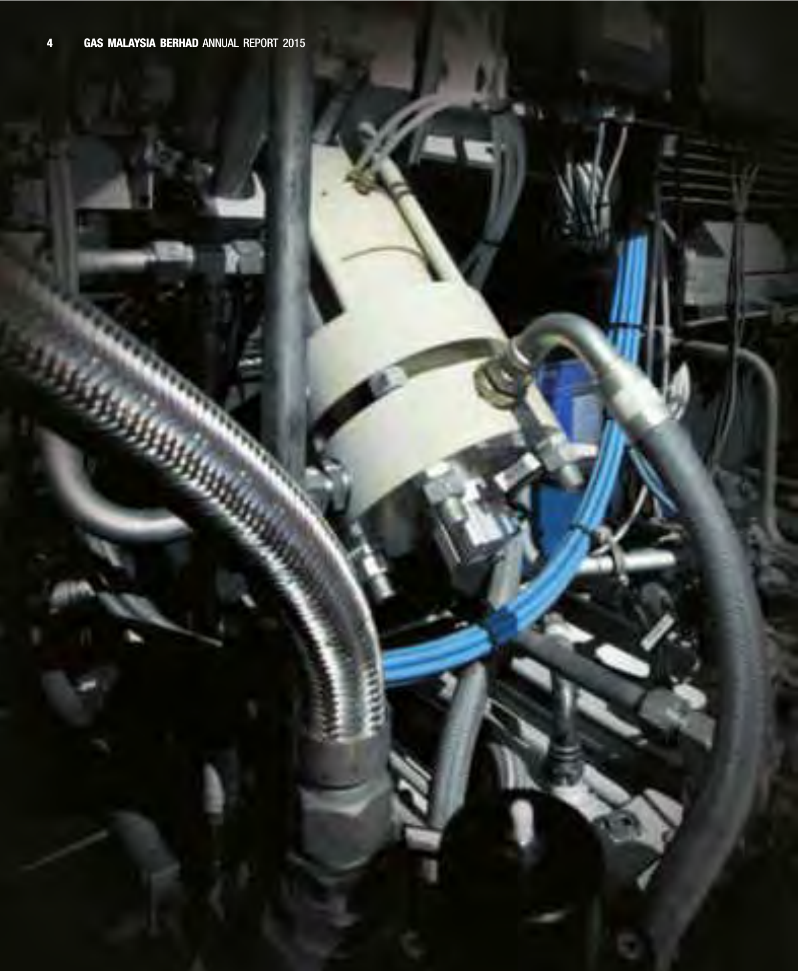
A component in Virtual Pipeline's mother station which compresses natural gas into the tube skid trailer.
