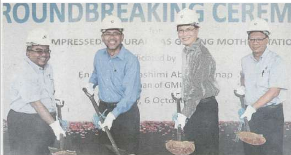
Ahmad Hashimi (second from left) and IEV Group CEO and president Christopher Nghia Do (third from left) officiating the groundbreaking ceremony in Kuantan recently
